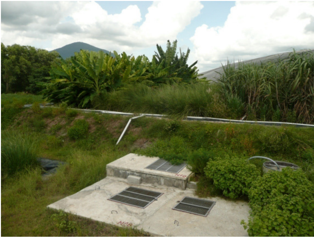
Constructed wetlands (OKA 3)
